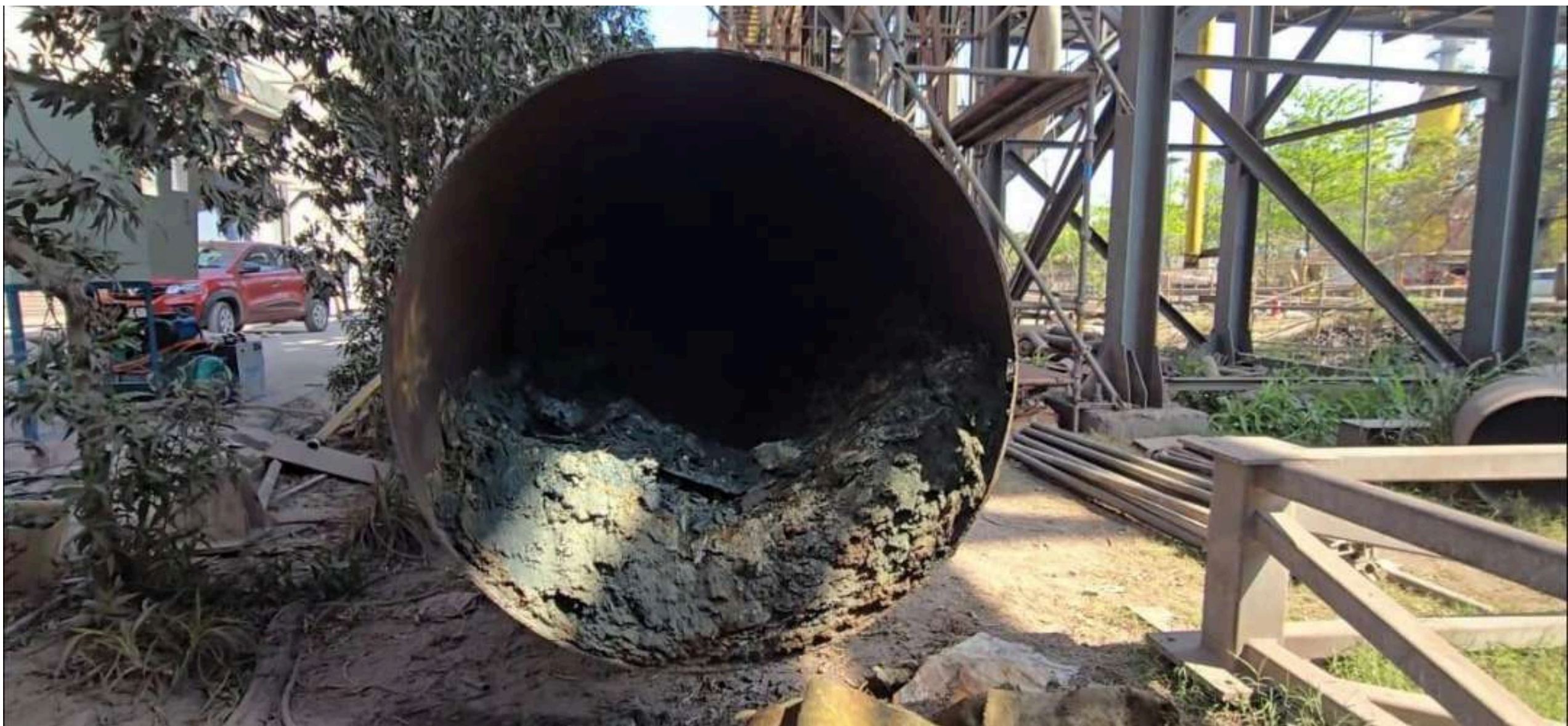
Fig.2: Slag Deposit in industrial pipe
